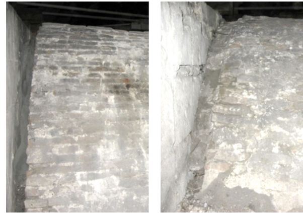
Fig. 5. The interface between the nave walls and vaults of (left) damaged and (right) undamaged vaults. The gap between the walls and vaults of the undamaged vault is filled with plastic sheets.
